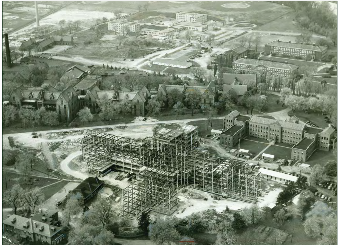
Figure III.44. Oblique aerial of the medical-surgical building under construction, circa 1950. The new patient facility was constructed over much of the open space available for patient recreation. Image courtesy Buffalo & Erie County Historical Society. (R-BRO-BHS-6a.jpg)
