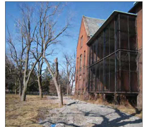
Figure IV.10. Many existing trees exhibit damage, likely as result of both compaction from the gravel construction drive and winter storm events. Courtesy HL. (R- BRO_20080403_0973.jpg)
